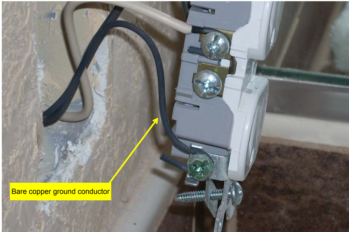
The bare copper ground conductor shows a heavy oxide coating
